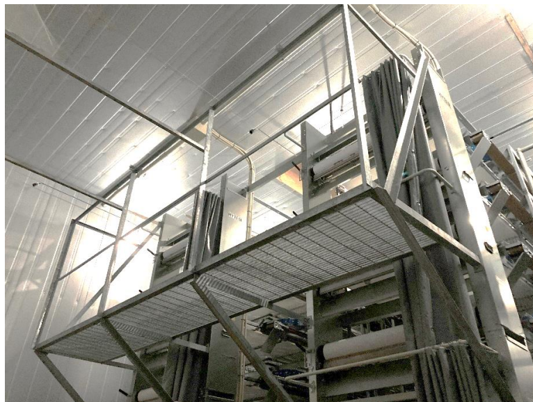
Working deck for Manure Collector
