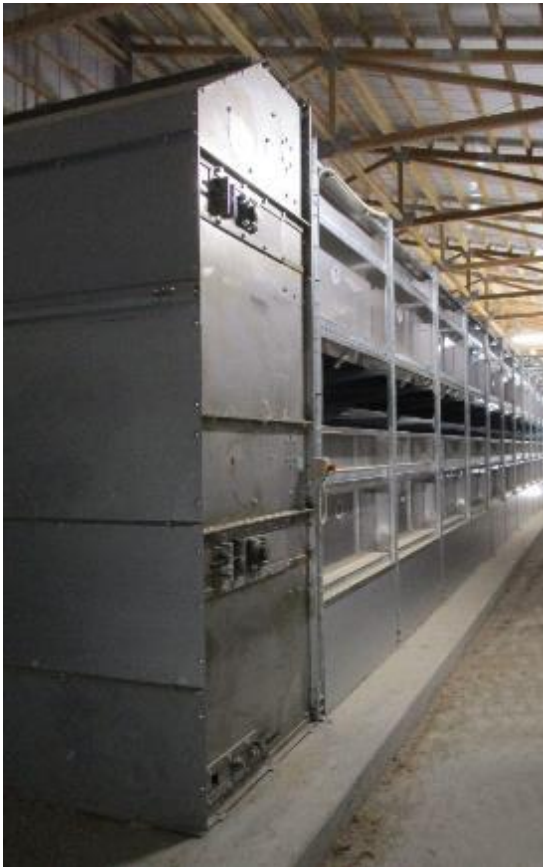
Out of four tiers, the top two tiers used for manure in higher water content is made of 304 stainless.
